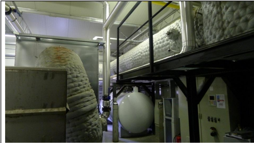
Horizontale buis rookgassen in ketelhuis
