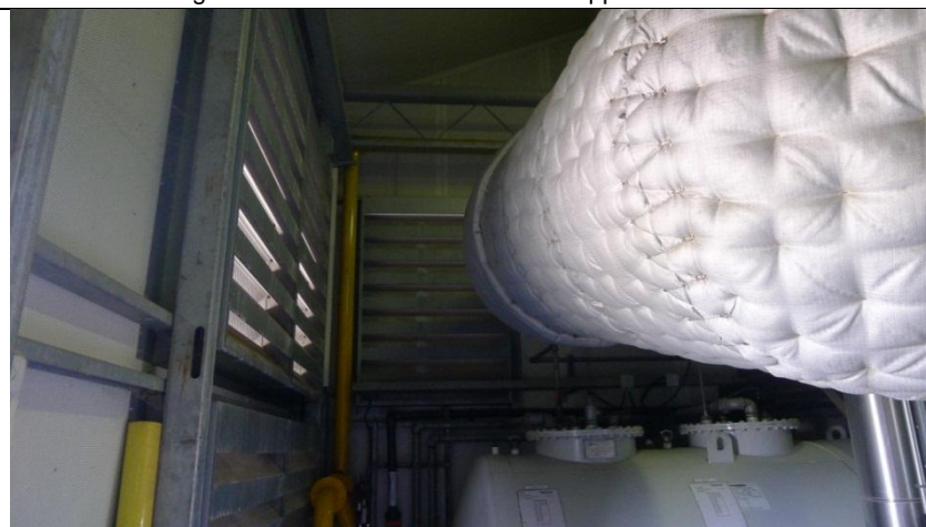
Horizontale buis rookgassen in ketelhuis, links ventilatieroosters
