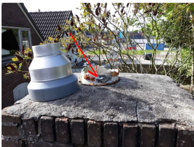
Foto 1: MM4, buis in schoorsteen
