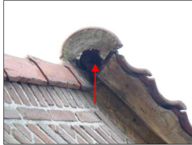
Figuur 21. Opening langs dakrand woning.
