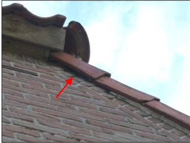
Figuur 20. Opening langs dakrand woning.
