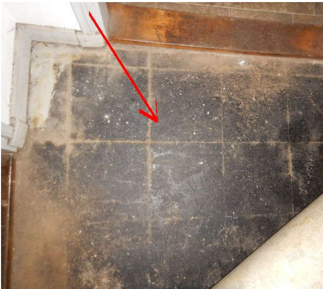
Bron 6, M05 bitumen (2)
