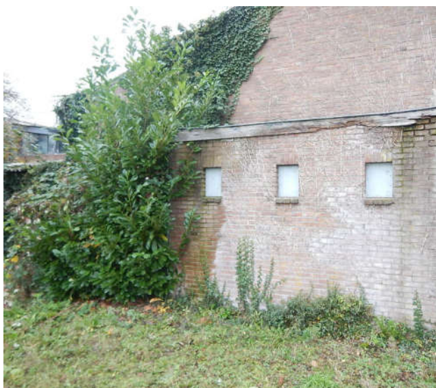
Bron 15, M14 bitumen (2)
