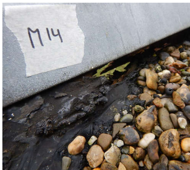
Bron 15, M14 bitumen (1)
