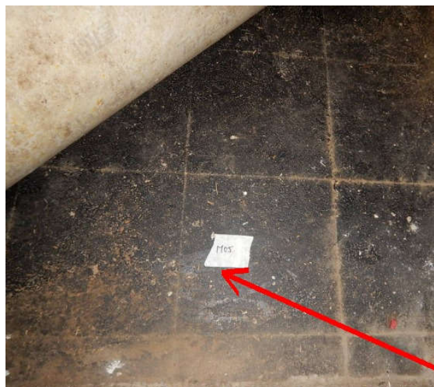
Bron 6, M05 bitumen (3)
