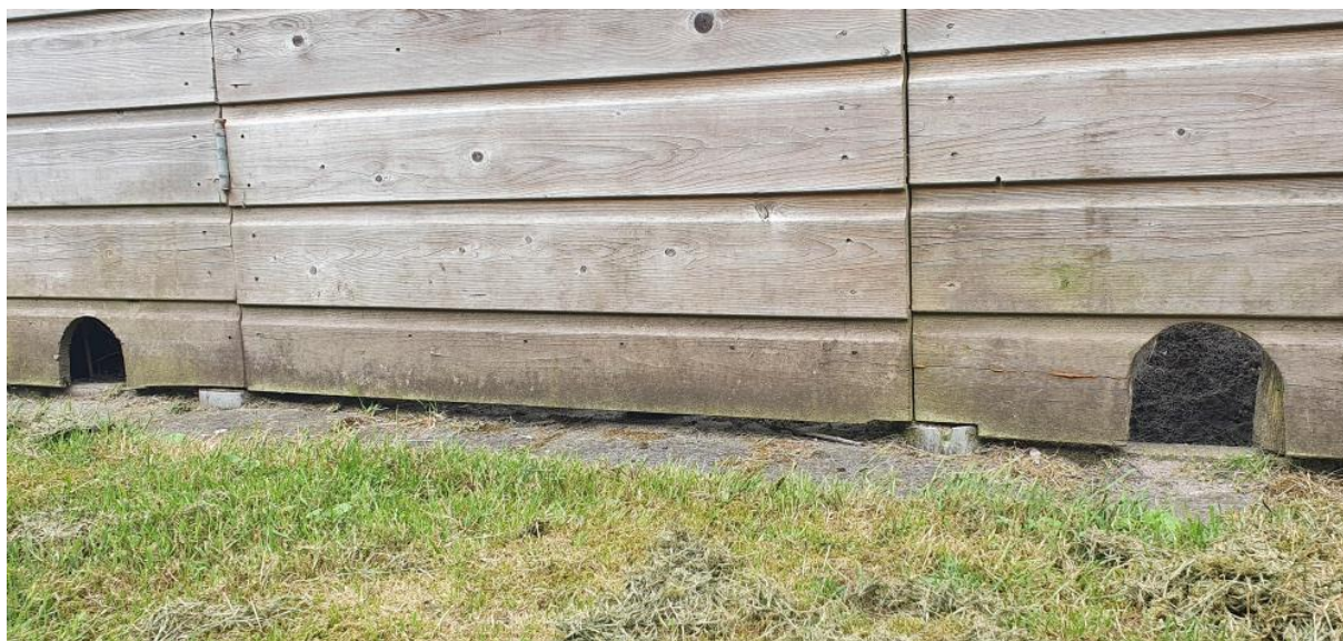
Figuur 17. Egelopening in schutting.
